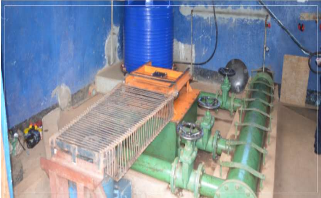
Figure 1-12. A photo showing inside Bondo 1 powerhouse where electro-mechanical equipment, mainly turbine and generator, are housed. (Source: Photo by the Author)
