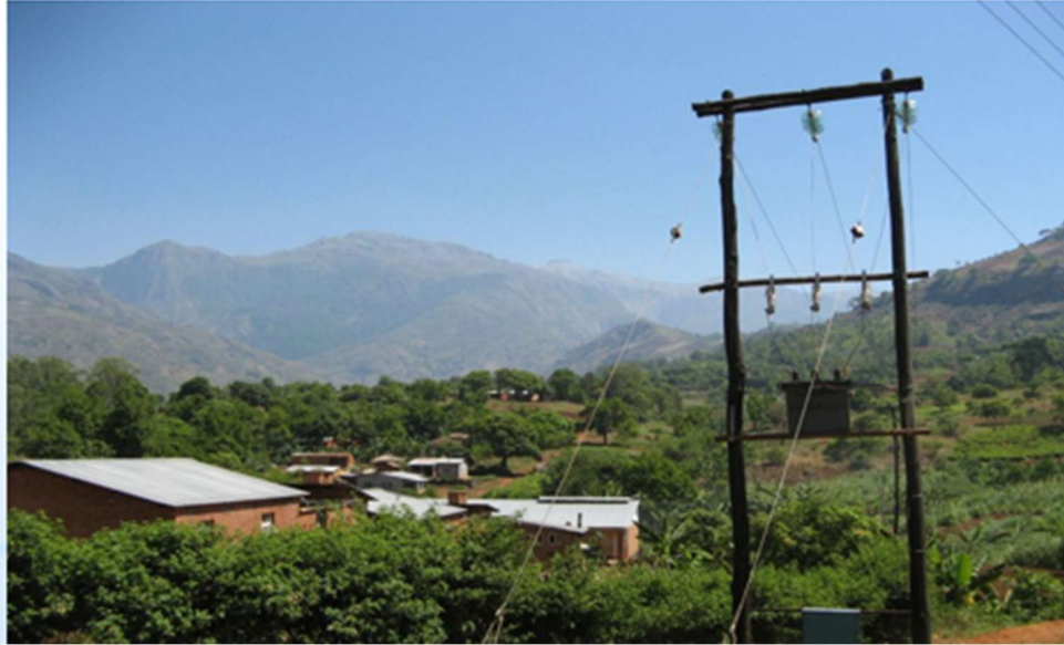
Figure 1-13. A photo showing a step-down transformer and the houses benefiting from the mini-grid. (Source: Photo by the Author)
