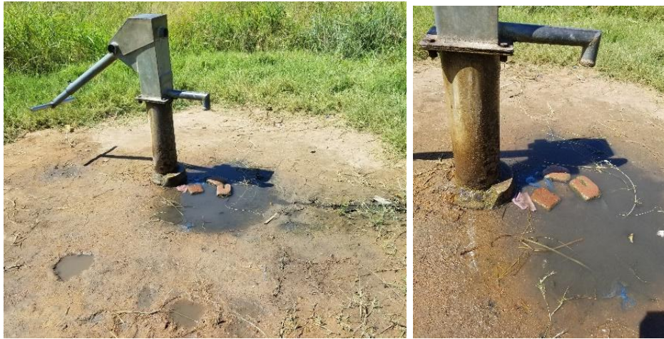
Figure 4-9: Borehole with no apron
