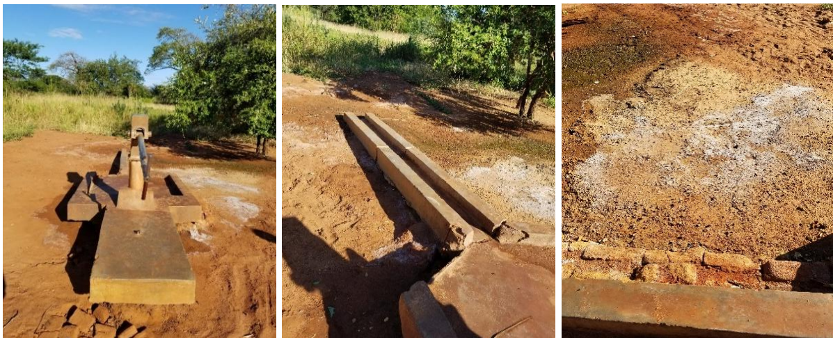
Figure 4-12: Whitish substance on ground surface as evidence of high salinity
