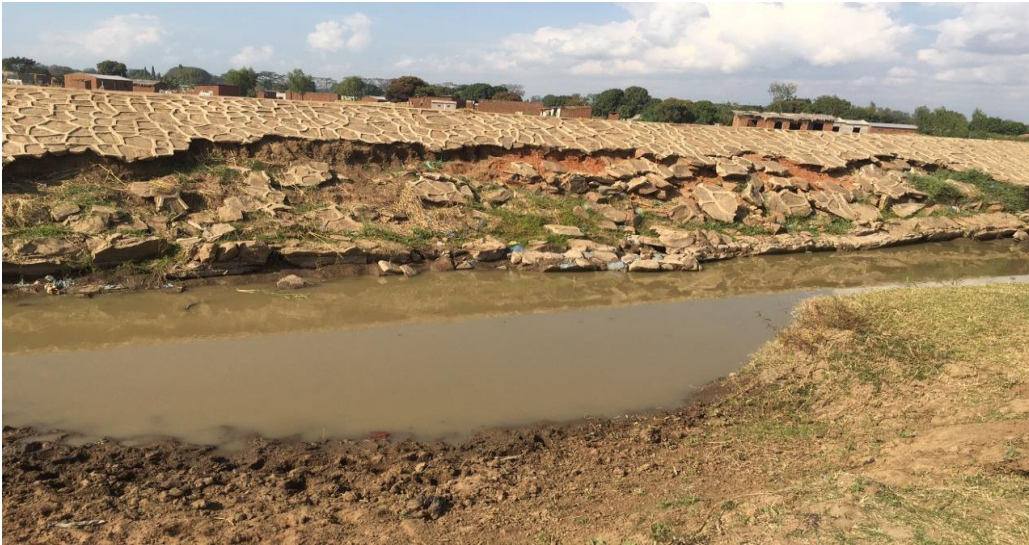
Figure 19: A dyke worn out by flood waters due to gullies created by brick molding and farming in 2023
