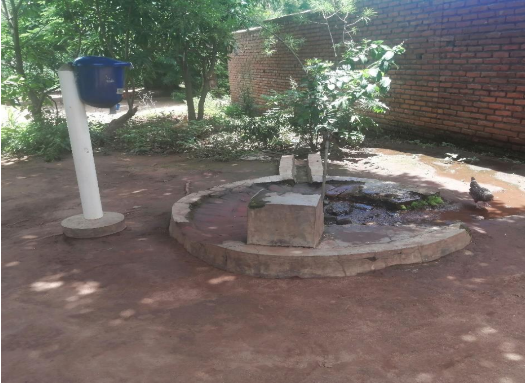
Figure 11: An installed chlorine dispensers through health projects
