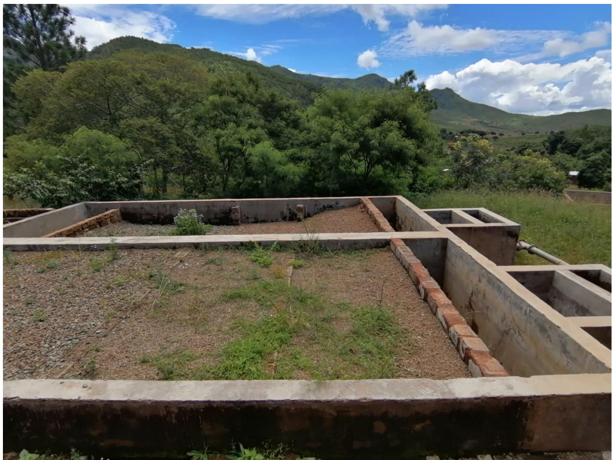
Figure 123: A defunct sand filter at Zomba East
