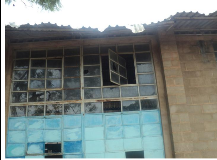
Figure28: Student G (15 years old): Broken window glasses and damaged roofing of a dining hall
