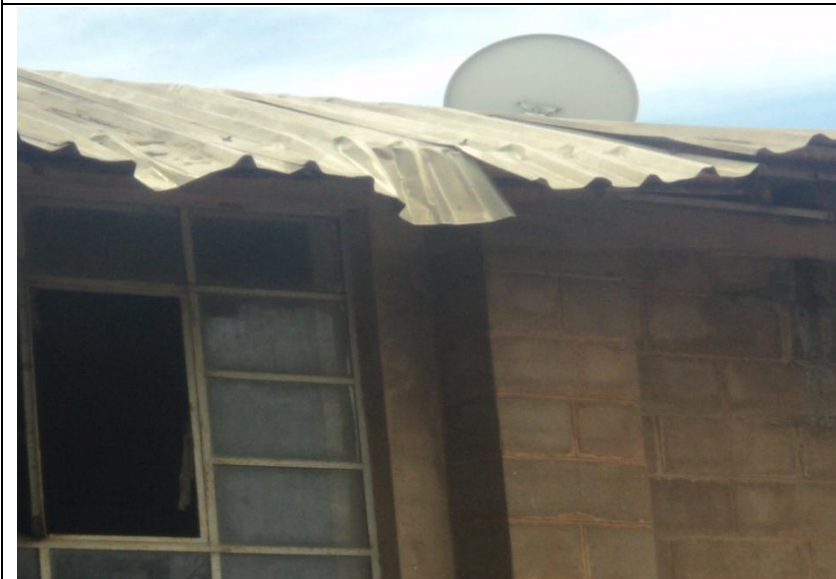
Figure12: Student H (16 years old): Damages done to window glasses, roofing and television satellite dish
