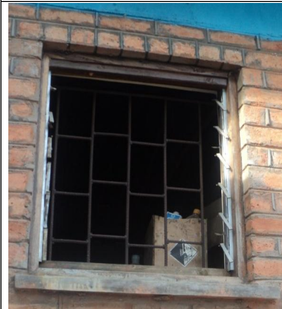
Figure 20: Student Y: ‘vandalism can be prevented through cooperation between teachers and students due to contacts and dialogue...’ photo showing broken window glasses of a laboratory
