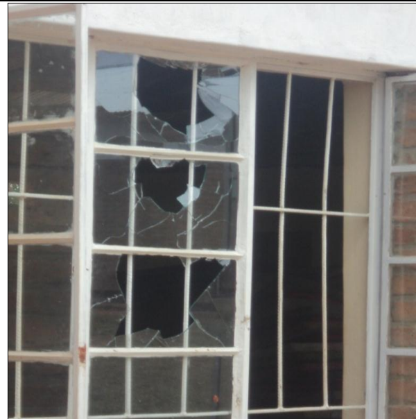
Figure 8: Student D: 'the many cause was lack of entertainment...' Photo showing broken window glasses of assembly hall.
