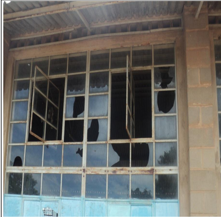
Figure 3: Student F (17 years old): “... calling students with stupid and meaningless names for example ‘mbuli’...” and also missing and reporting late for classes. Photo showing unreplaced broken window glasses from 2010 to 2014.
