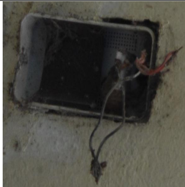
Figure 14: Student P: One of the damaged security bulbs.
