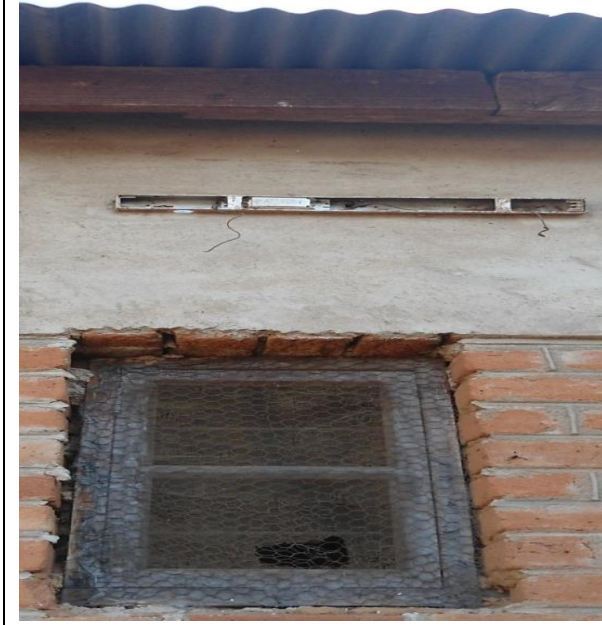
Figure 22: Student R: Wire mesh replacing window glasses which were blocken but also a security bulbs at the hedmaters office.
