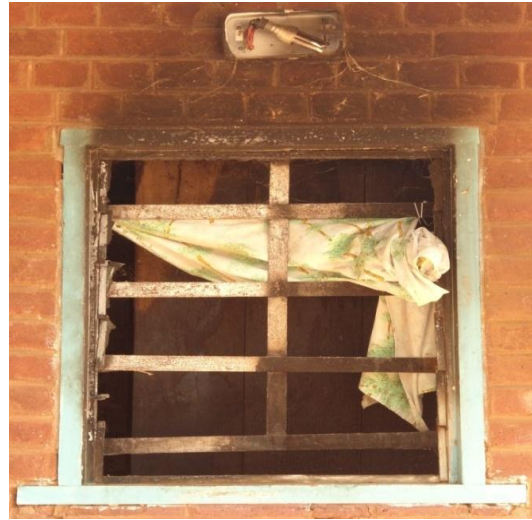
Figure 1: Student L, 15 years old : photo showing broken security bulb and window glasses
