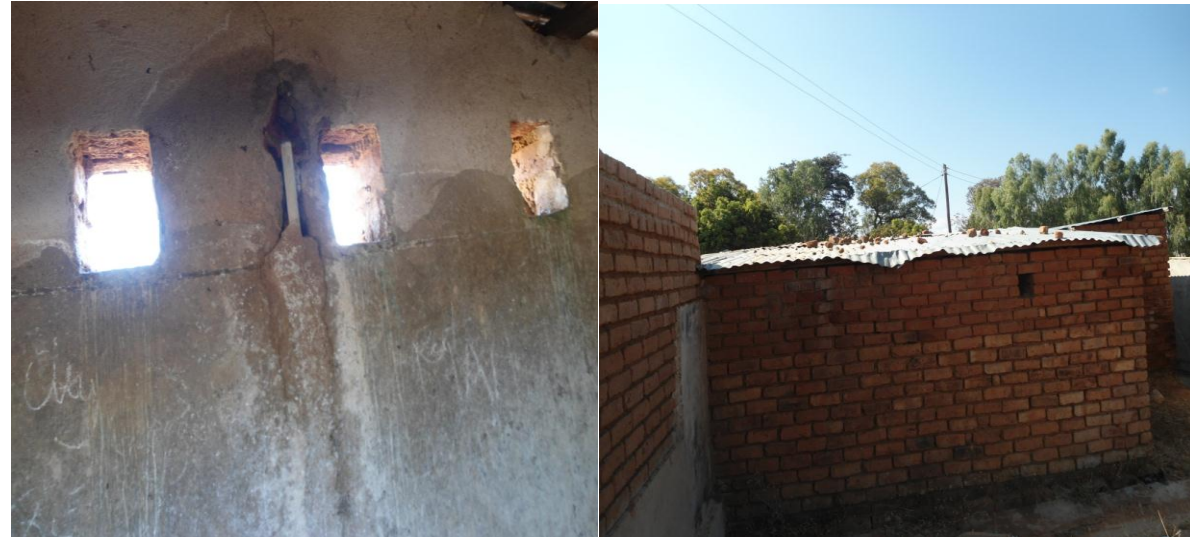
Figure 18: Student S: vandalised water pipes inside Boys bathrooms and stones on top of a toilet block. Some suspected students were expelled from school.
